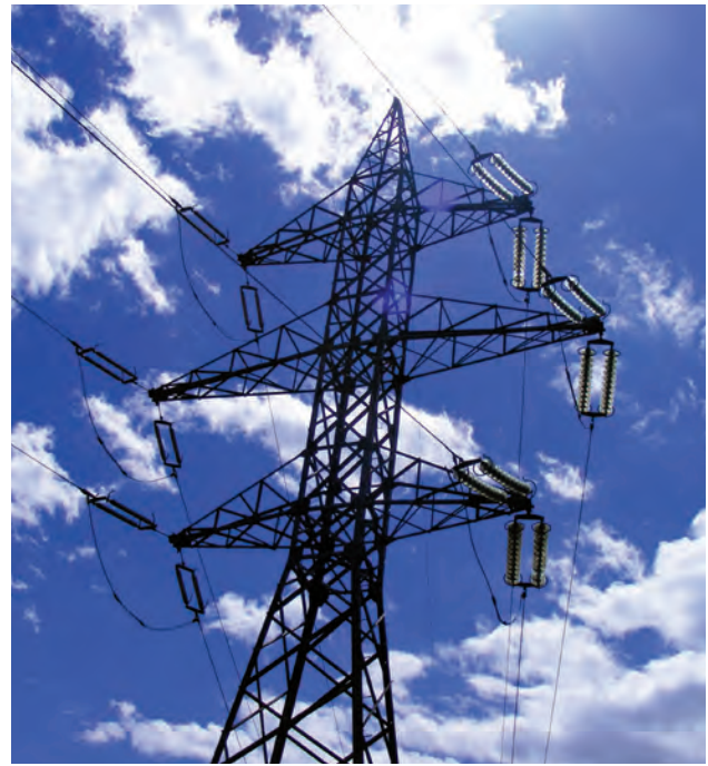
Electricity transmission wires. Photo credit: Emilian Robert Vicol, Pixabay
