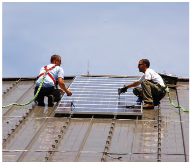
Fort Dix solar panels. Photo credit: U.S. Army Environmental Command
