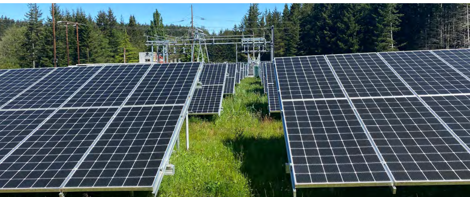
Solar installation at the Decatur Island Community Solar Project. Orcas Power & Light Cooperative
