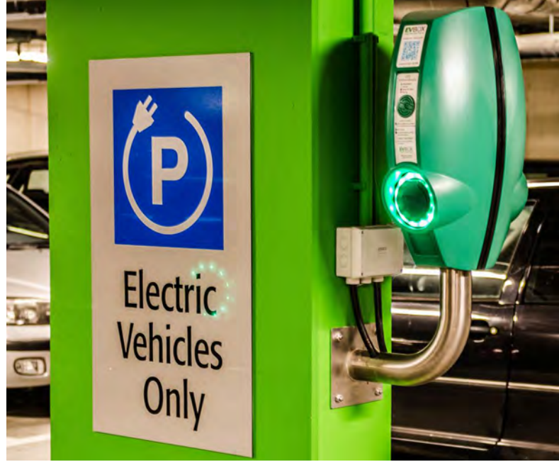
EV charging station. stanvpetersen
